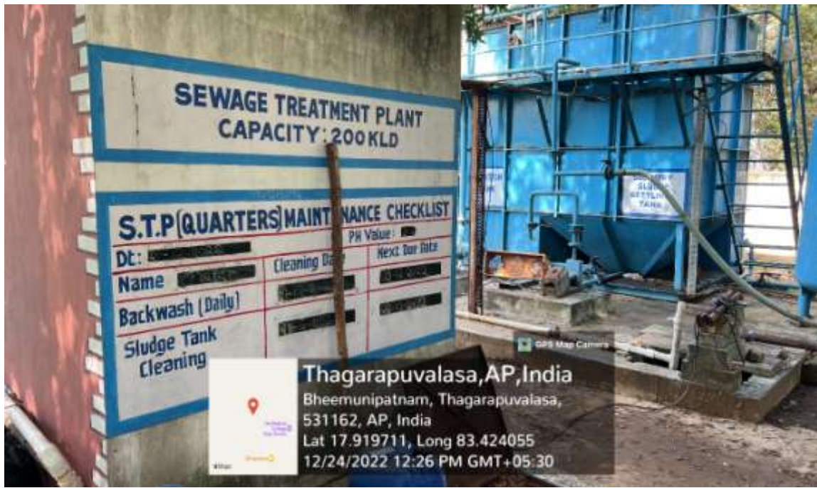
Waste water recycling plant
