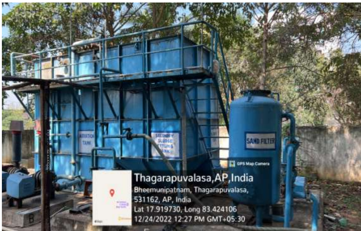
Waste water recycling plant
