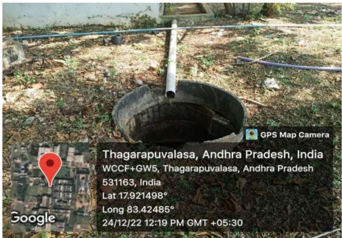
Bore well /Open well recharge
