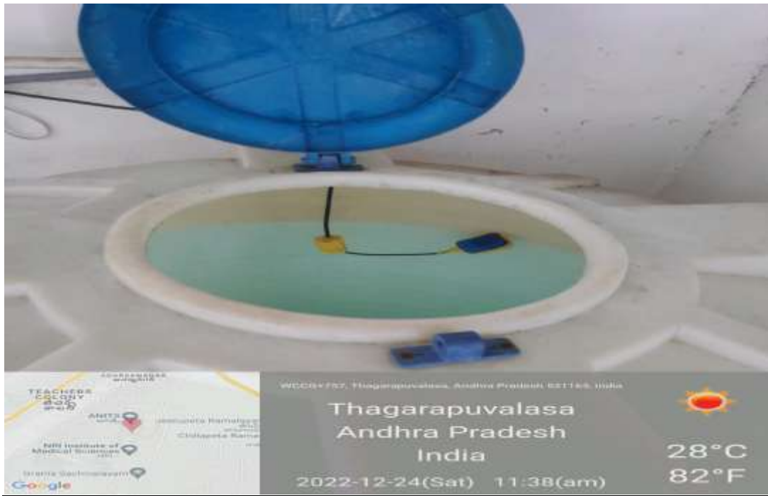
Electric sensor at F-Block RO plant for automatic switch on and off pump
