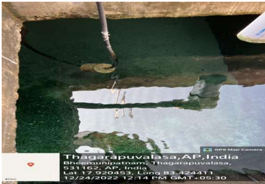
Electric sensor at H-Block rooftop tank for automatic switch on and off pump
