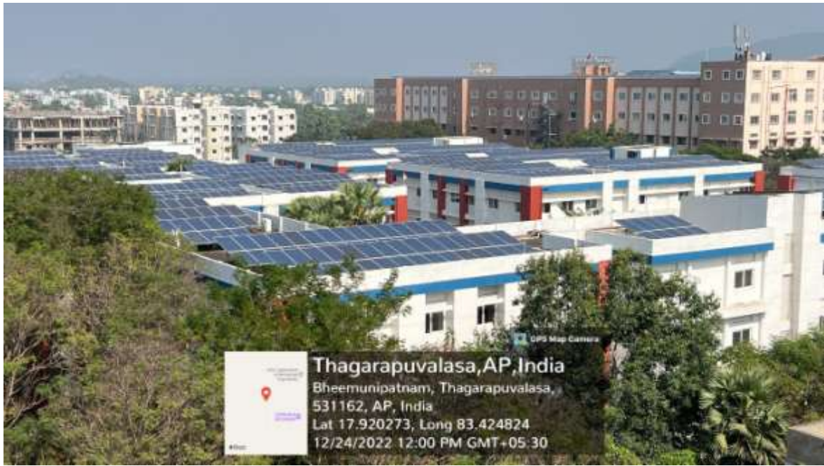
Rooftop solar panels on all buildings in the campus
