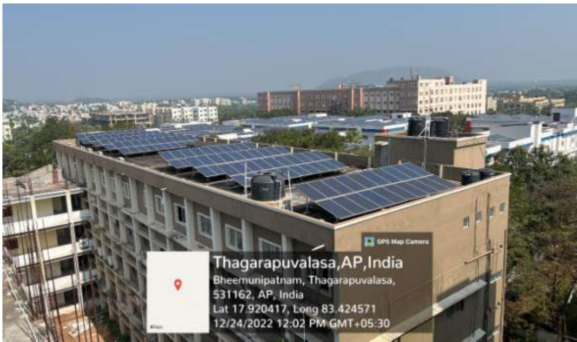
Rooftop solar panels on all buildings in the campus
