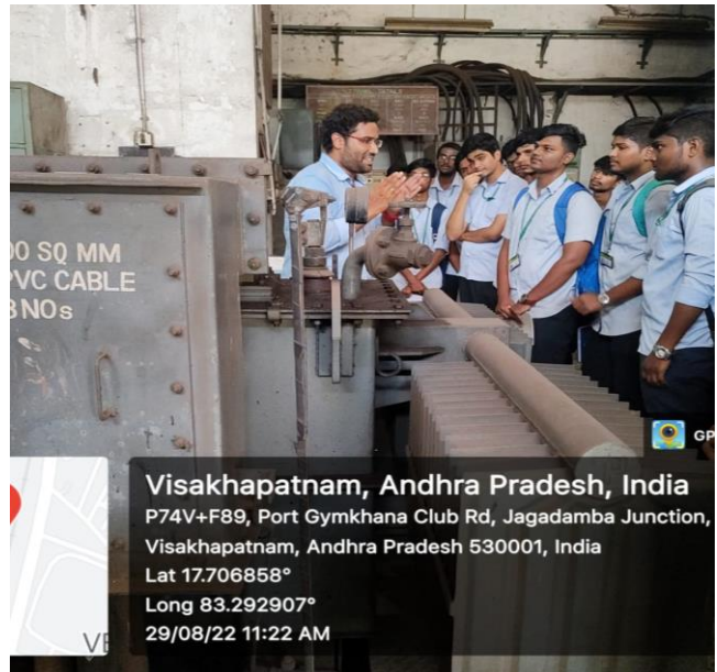
Fig 5: Technical expert explaining working of the transformer on how it was managed with excessive load attached and precautionary steps to deliver the power requirement of industry.
